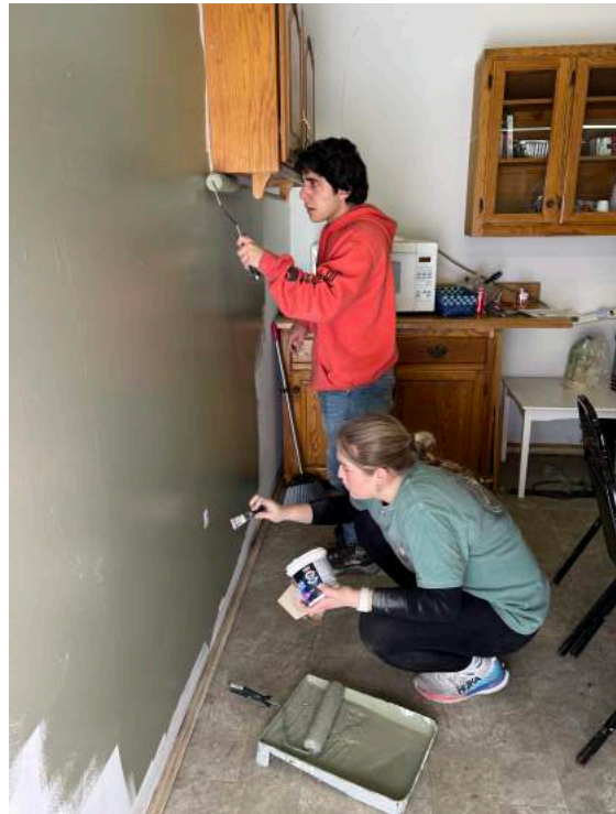
Christian and Katie freshen up the Habitat ReStore with a fresh coat of paint
